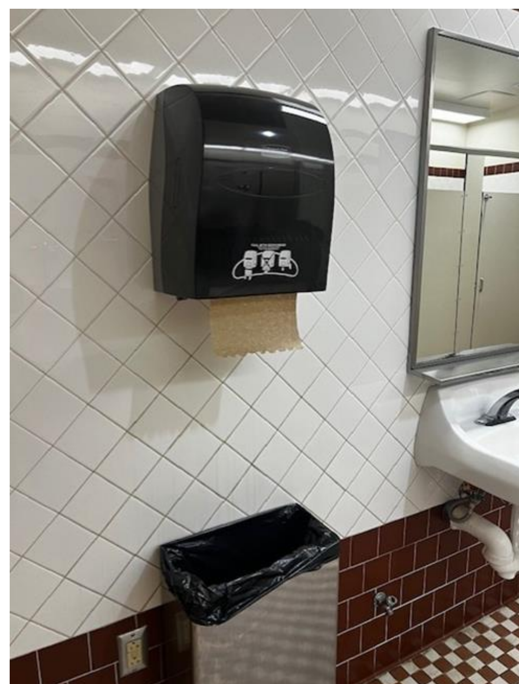
Figure 1: Photo of men's SURC west bathroom prior to DYSON Airblade V installation.
