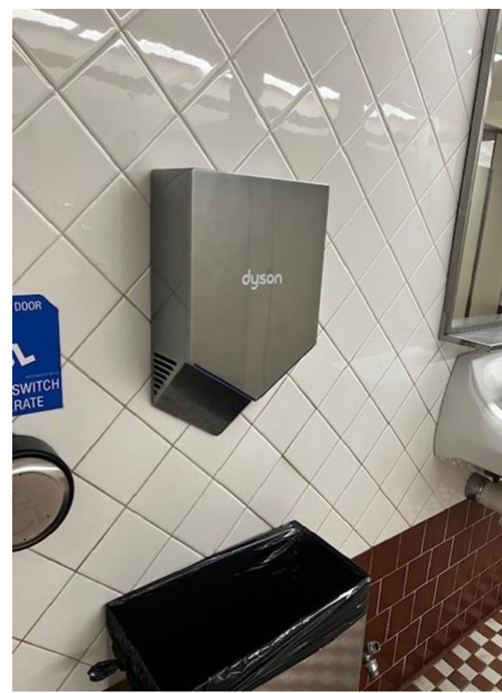
Figure 3: Photo of men's SURC east bathroom after DYSON Airblade V Pilot installation.
